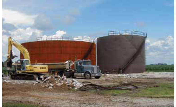
StateLine Cooperative's Armstrong location received special attention from a road grader earlier this summer to accommodate the new liquid fertilizer loading facilities and liquid fertilizer equipment expansion. The two tanks were added within the last two years.
