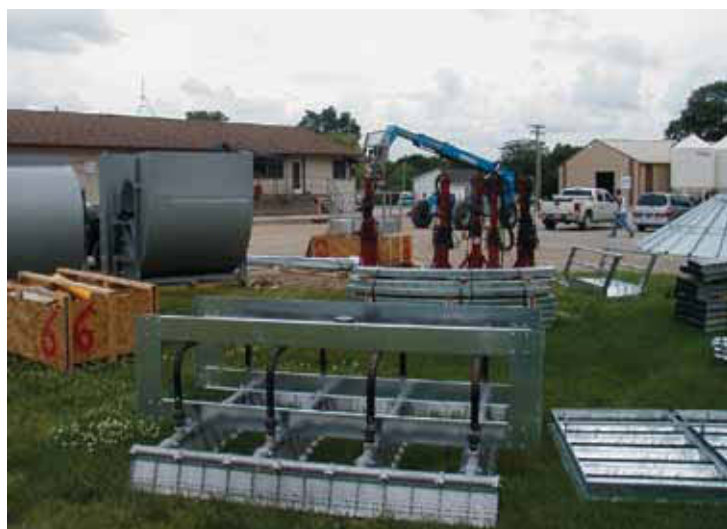
At StateLine Cooperative's Ringsted location, a new continuous flow natural gas dryer is being built to provide increased drying capacity system-wide.
